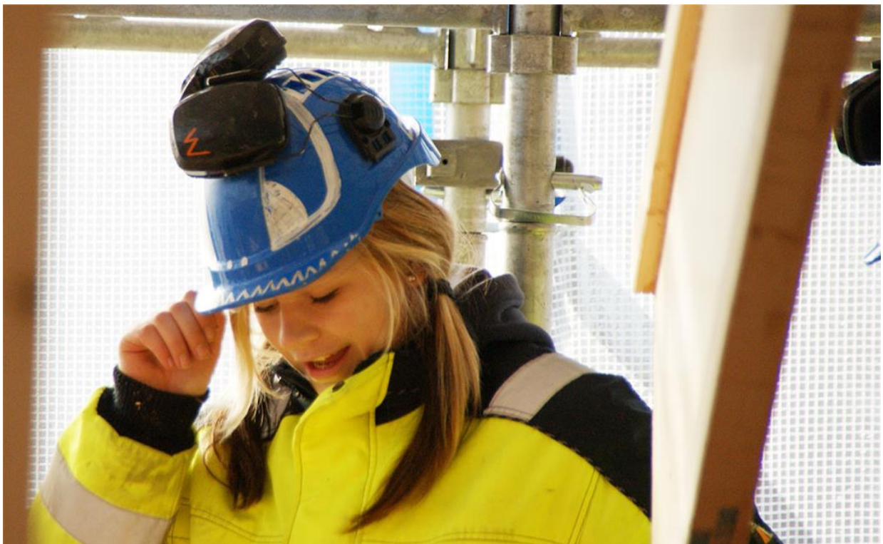
Figure 1C4. Students are building the northern-most single family houses certified to passive house standard. To meet future energy regulations it's important to educate craftsmen with the know-how and workmanship needed to go the extra mile.
